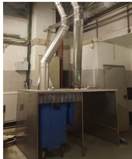
Newly designed waste chutes for food waste in CascaiShopping
